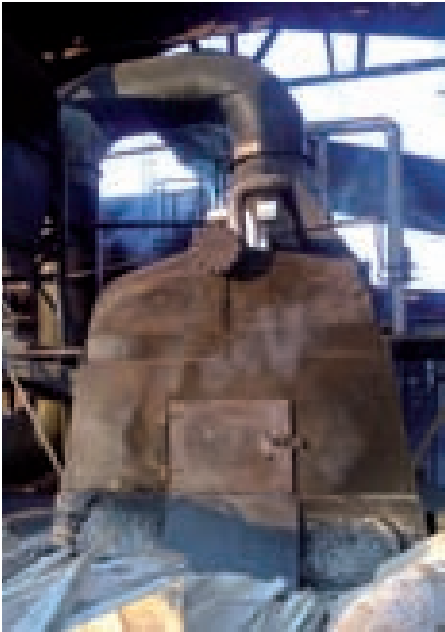
Furnace for generating electricity
